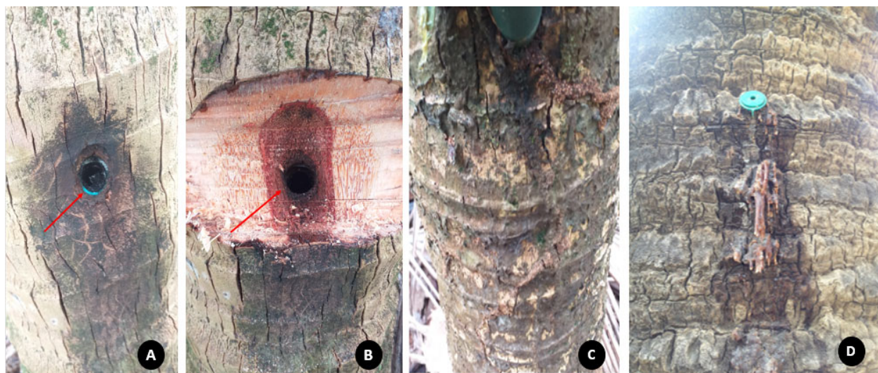
Figure 11. Fixation of catheter/pipe in palm stem. (A–C) Vita Caule® catheter/pipe break, port exposure, and damage to the coconut stem. The red arrow at A indicates that the catheter/pipe was broken inside the stem, and in B, the other palm with an area of damaged vascular bundles using this permanent accessory; (D) Exudation of the palm stem using SOS Palm®. Source: Collection of the authors' pictures.
