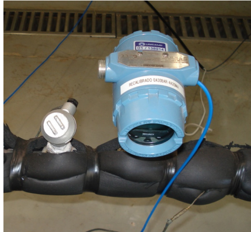
Figure 3.5. Pressure gauge and thermocouple in the inlet of the pipeline (Luthi, 2013).
