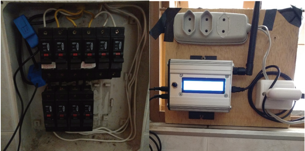
Figure C.4: Open source smart meter installed locally for experiments
