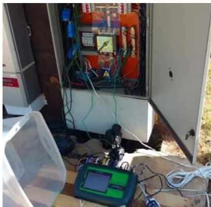
Fig. 4 Energy meter connected to the output of a three-phase solar inverter in Tanquinho solar power plant, Brazil
