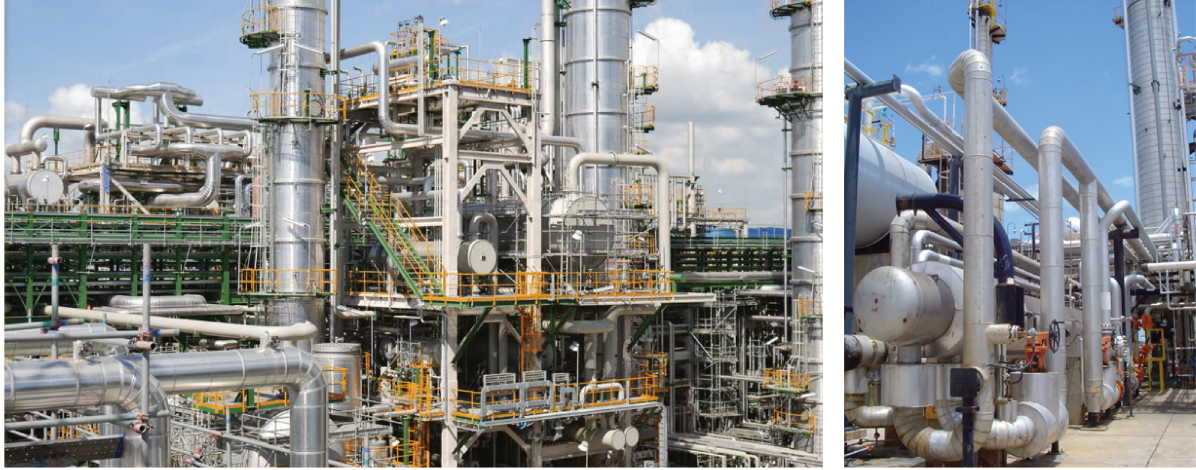
Figure 1 – Examples of complex geometries with the presence of different object scales and congestion.
